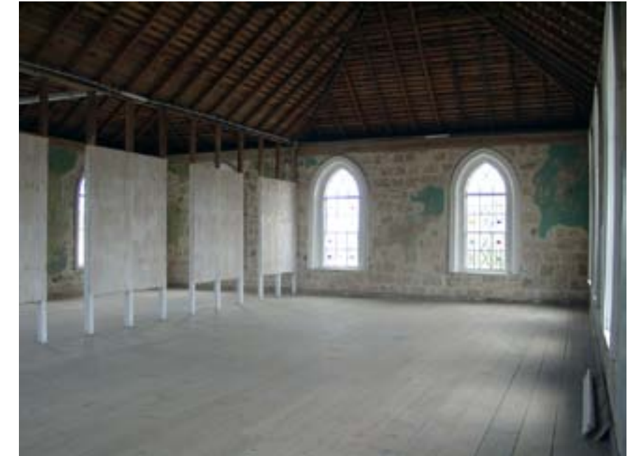
The roof framing system on the interior of the Baptist Manse (c. 1798) is left completely exposed to help cool the inside.
