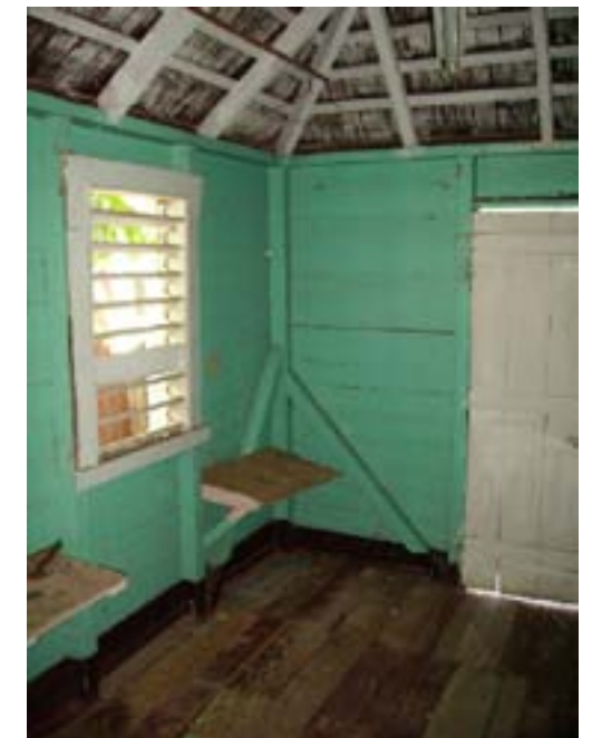
The inside of this small board house also has an exposed roof system to promote greater air circulation.
