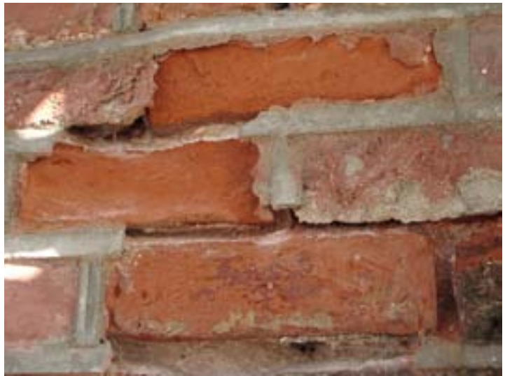
This house had been damaged by the application of Portland cement in the mortar joints, which trapped moisture in the bricks and caused the faces to deteriorate and pop out.
