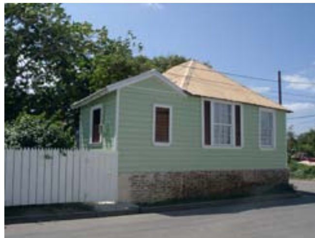
Above: 7A Lower Harbour Street was restored and the original brick pier foundation was stabilized and kept in place to promote ventilation underneath the structure. Below: The original foundation at 3 Lower Harbour Street was also maintained and preserved.
