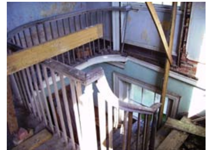
Above: A wood frame house in need of repair. Below: a wooden staircase being renovated at 21 Duke Street.
