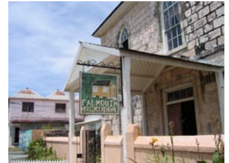
The entrance door restoration at the historic Baptist Manse kept the original double wooden door and opening, and maintained the transom light above.
