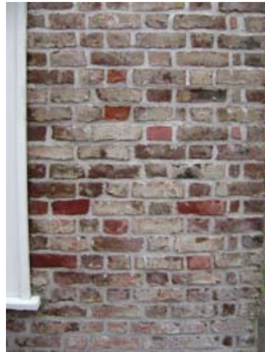
Above: Deteriorated brick caused by the use of incompatible Portland cement in the mortar joints. Below: A brick building repointed with an appropriate lime-based mortar.
