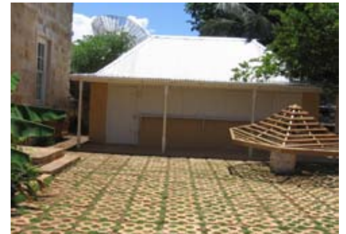
Above: The rear of a building near Water Square in need of decorative elements outlined in the guidelines. Below: An appropriate rear courtyard restoration.
